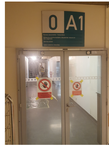
(e) A corridor of the ground floor is being renovated. Access to the other end of the corridor is available only by going outdoors or through another floor.
