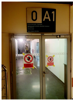
(e) A corridor of the ground floor is being renovated. Access to the other end of the corridor is available only by going outdoors or through another floor.
