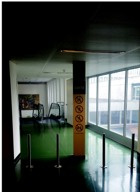
(c) Warning sign before an escalator leading to the exit, mentioning that it is not suitable for people using a cane or a wheelchair. No alternative root sign exists though.
